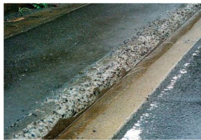
Fig.2 Salt Scaling of Concrete due to the Influence of the Deicing chemicals
