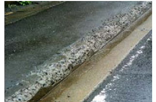
Fig. 1 Scaling damage to concrete products.
