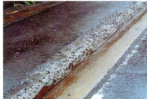
Fig.2 Salt Scaling of Concrete due to the Influence of the Deicing chemicals
